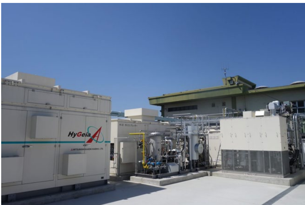
Fukuoka City hydrogen production facility
