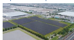
Japan's largest-scale captive-consumption solar power system (Gunma Oizumi Plant)
