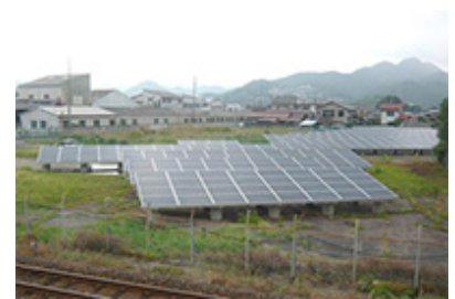
Solar power generation system with the output corresponding to the use by 100 detached houses.
