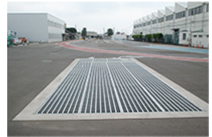
Flood prevention measure (drainage grid) (Utsunomiya Plant)
