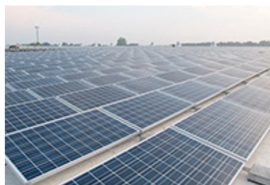
1 MW Power Generation Facility
