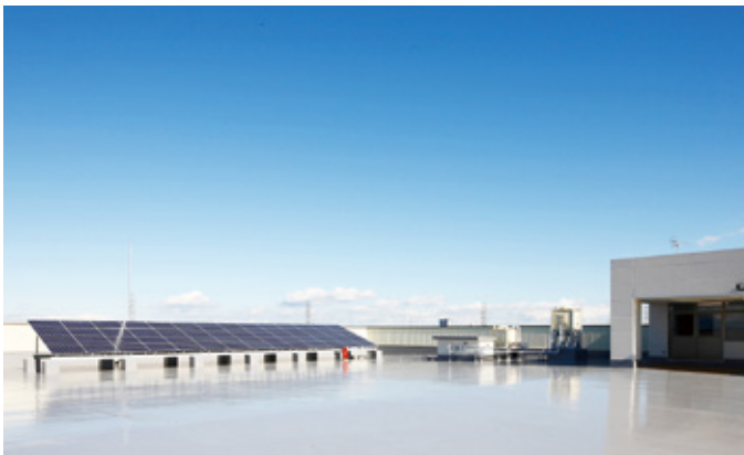
Solar power cells installed on the roof of the new administration building
