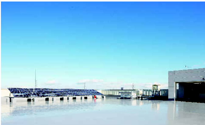
Solar power cells installed on the roof of the new administration building
