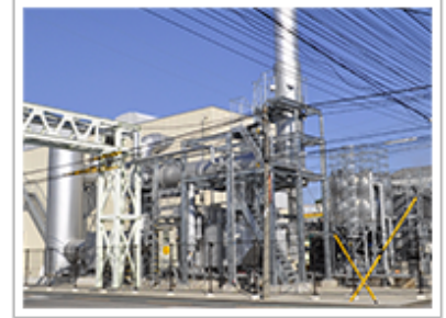
Gunma Manufacturing Division The Main Plant's cogeneration system
