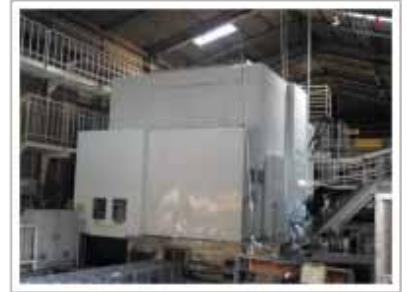
Baler press noise insulation
