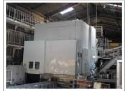
Baler press noise insulation
