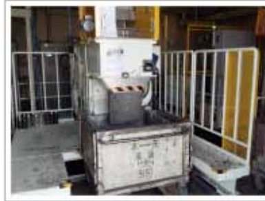
Paint dregs recovery equipment
