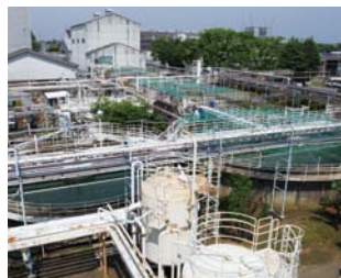
Wastewater treatment system
