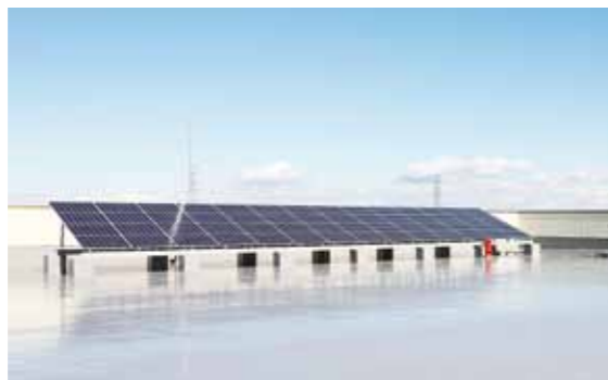
Solar power cells set on the roof of the new administration building
