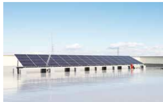
Solar power cells set on the roof of the new administration building
