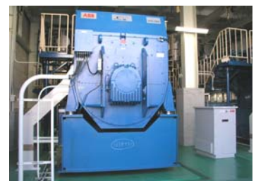
Natural gas cogeneration systems at the Oizumi Plant
