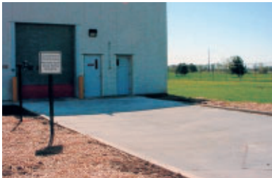
The concrete cover installed in front of the paint solvent recovery facility
