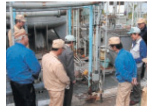
Checking the pH meter and the level sensor.
